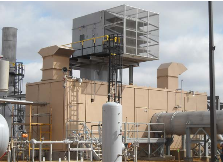
GAS TURBINE ENCLOSURE
