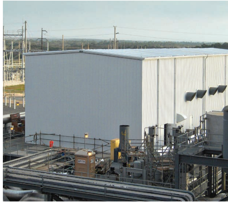
STEAM TURBINE ENCLOSURE
